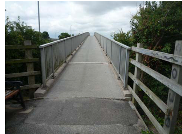
Pedestrian footbridge with no handrails
