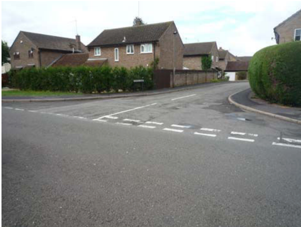
Example of road junction with no dropped kerbs or tactile warning
