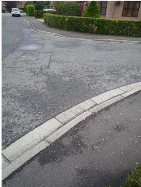
Dropped kerb location with no tactile warning
